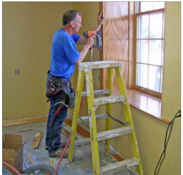
Contractor Joe Herter works his magic during the Gift Shop remodeling project.
